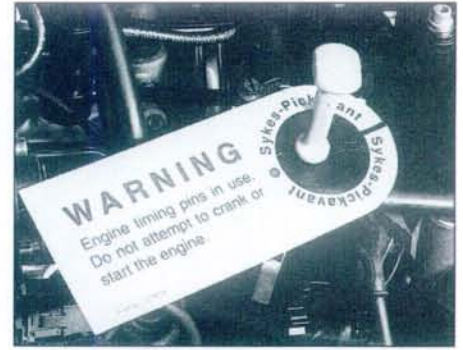
3.7 Warning notice in place in (typical) engine compartment
