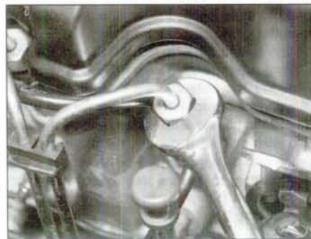
12.11a Unscrew the union nuts securing the injector pipes to the injectors . . .
